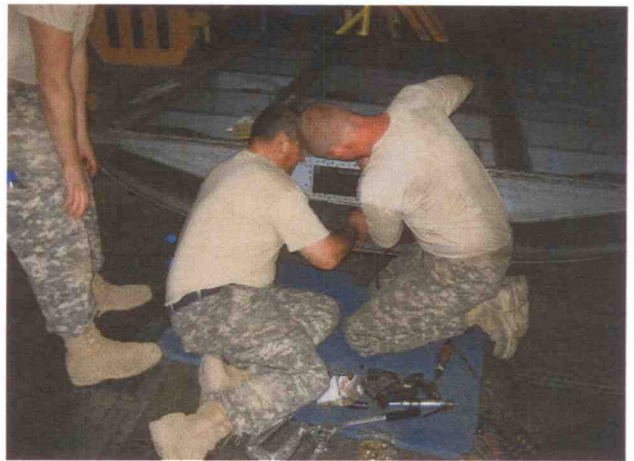
Senior Structural repairers SSG Rick Consdorf and SGT Jonathan Malone waste no time and go to work on the ramp repair as sheet metal apprentice SPC Robert Johnson looks, listens, and learns.
